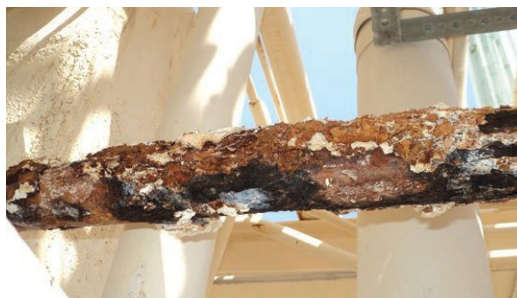
Significantly more corrosion was found during inspection.
