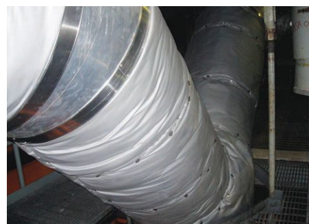
Energy costs can be reduced by millions of dollars by improving insulation.
